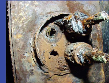
Severely corroded anchor head showing strand slippage and protective cap loss after 30 years in service
