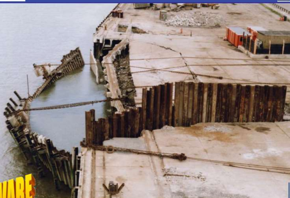
Anchored quay wall failure, River Thames
