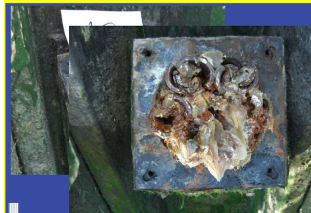
Corrosion induced fractured barrel and wedges and strand slippage after 11 years in service
