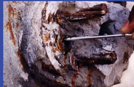
Severely corroded strand exhibiting slippage through wedges after 18 months in service
